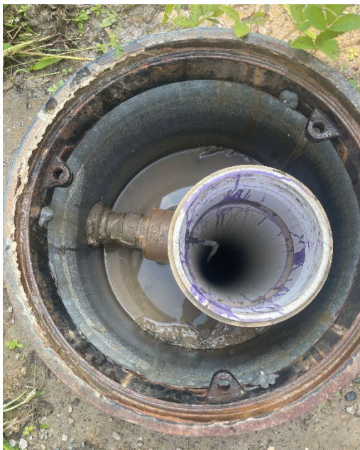
Figure 5. The 40T posthole instruments were deployed in cased holes to depths of down to 10 metres
