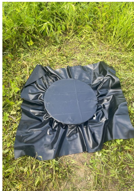
Figure 6. The cased holes were then sealed with tarpaulin and covered in mulch to protect against moisture ingress
