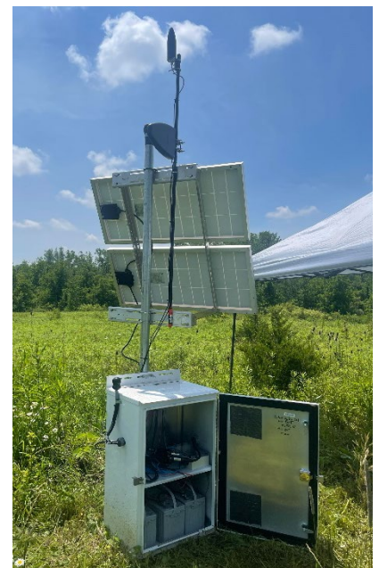
Figure 7. Stations are equipped with solar panel charged batteries to power the 40T Posthole and the Minimus digitiser, and with a cell modem to transmit the data to the network
