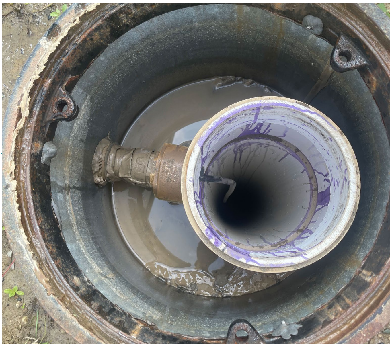
Figure 1. 40T Posthole instruments were deployed in cased holes to depths of up to 10 metres
