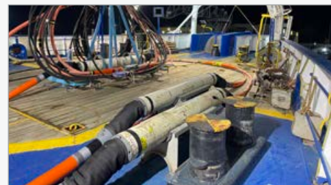
Image 8 : Top - Winching equipment from dockside onto the Antonio Meucci Image 9 : Bottom - The third repeater being placed onto the deck of the Antonio Meucci
