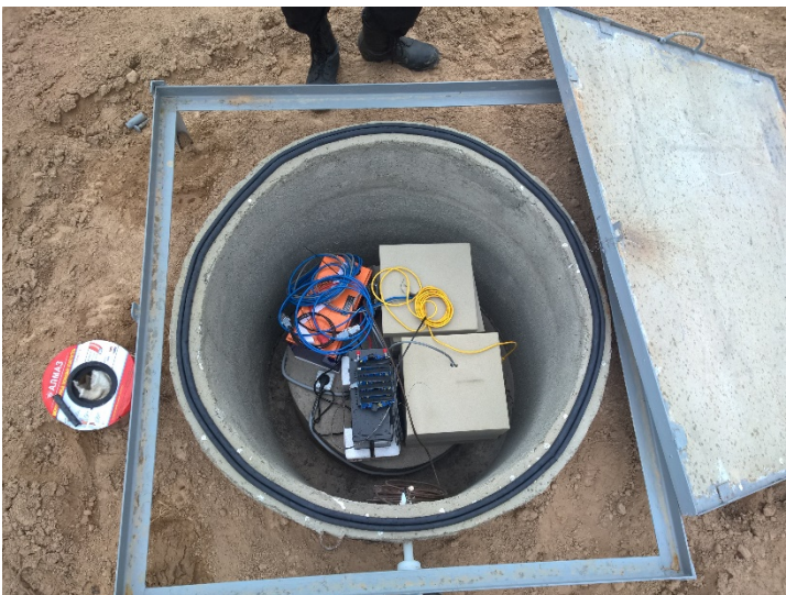
Figure 4. Example of a pit with Güralp products installed.
